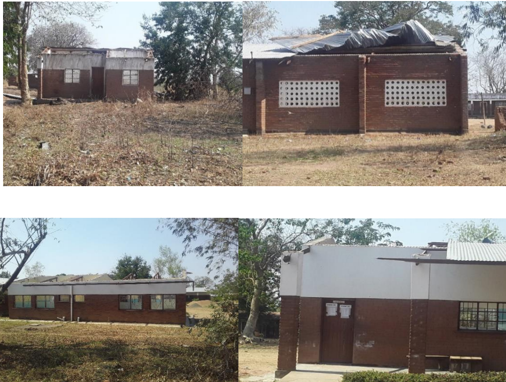
Figure 13: Strong Winds Blew off Roofs of Structures at Kapire Primary School and Kapire Community Day Secondary School (Kachenga Area) at the Beginning of 2020/2021 Rainfall Season.
